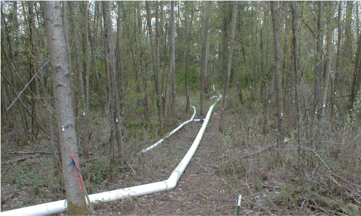
Figure 3 - 26: Manifold and Branches in a Wooded, Vegetated Spray Field
